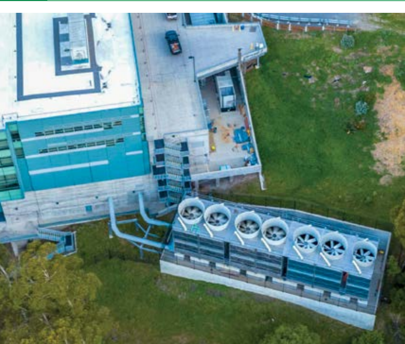
Figure 9. The NERSC cooling towers next to Shyh Wang Hall on the Berkeley Lab campus.
